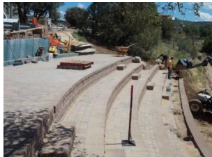
Centerfield plaza: A new centerfield plaza at the baseball park on the Prescott campus was constructed in 2013-14. Cost unknown.
